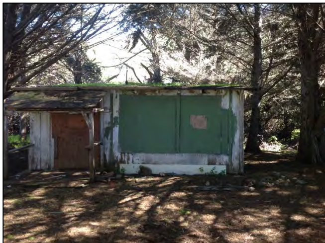
Photo 8: Unused cabin near the landslide area
