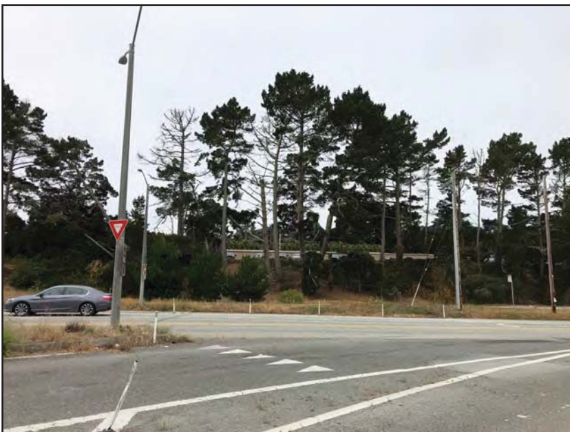
After demolition of existing buildings, construction of new building and removal of trees
